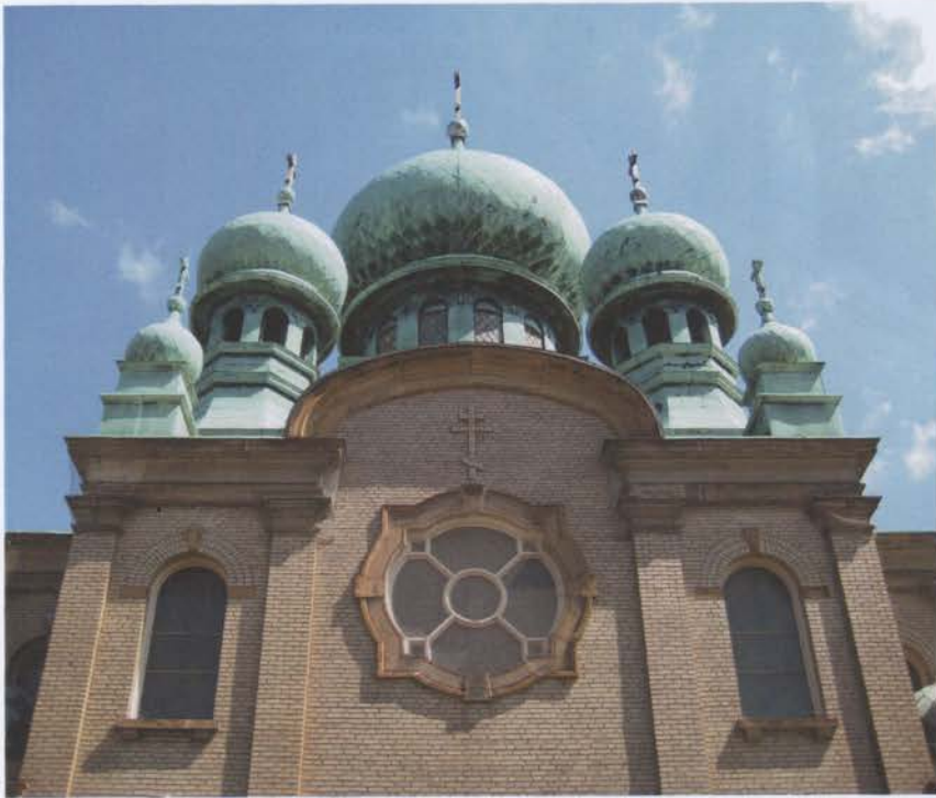
HOUSES OF THE HOLY AIC's project portfolio includes work on numerous religious structures, such as masonry façade and window restoration at the distinctive St. Theodosius Cathedral, a prominent presence in Cleveland's Tremont neighborhood.
